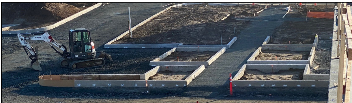
Bottom left: Forms are in place for curbs around landscape areas in the parking lot.
