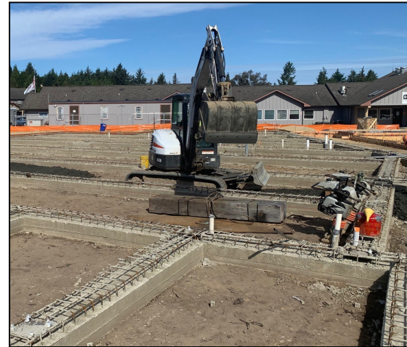
Left: An excavator spreads rock to fill the space between reinforced concrete “grade beams.” The beams and the rock fill between them will support the slab.
