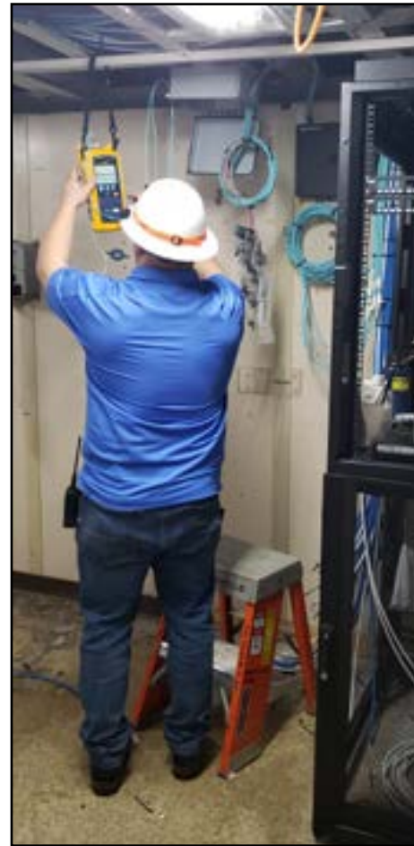
Tyson Cochran works below deck of an Army Corps of Engineers dredge, testing cable for final certification. The Tribal One team upgraded the entire communications systems for two dredges.
