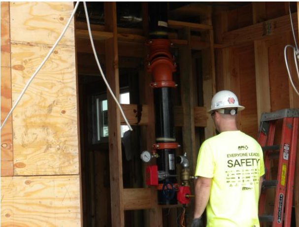
Fire riser room.
